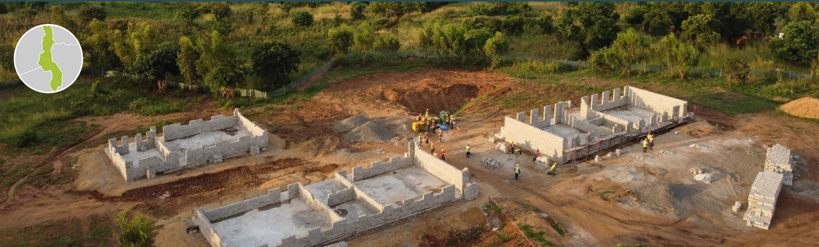
Malawi construction of rural SEED community day secondary school © 2022 Matt Harder/Tetra Tech
